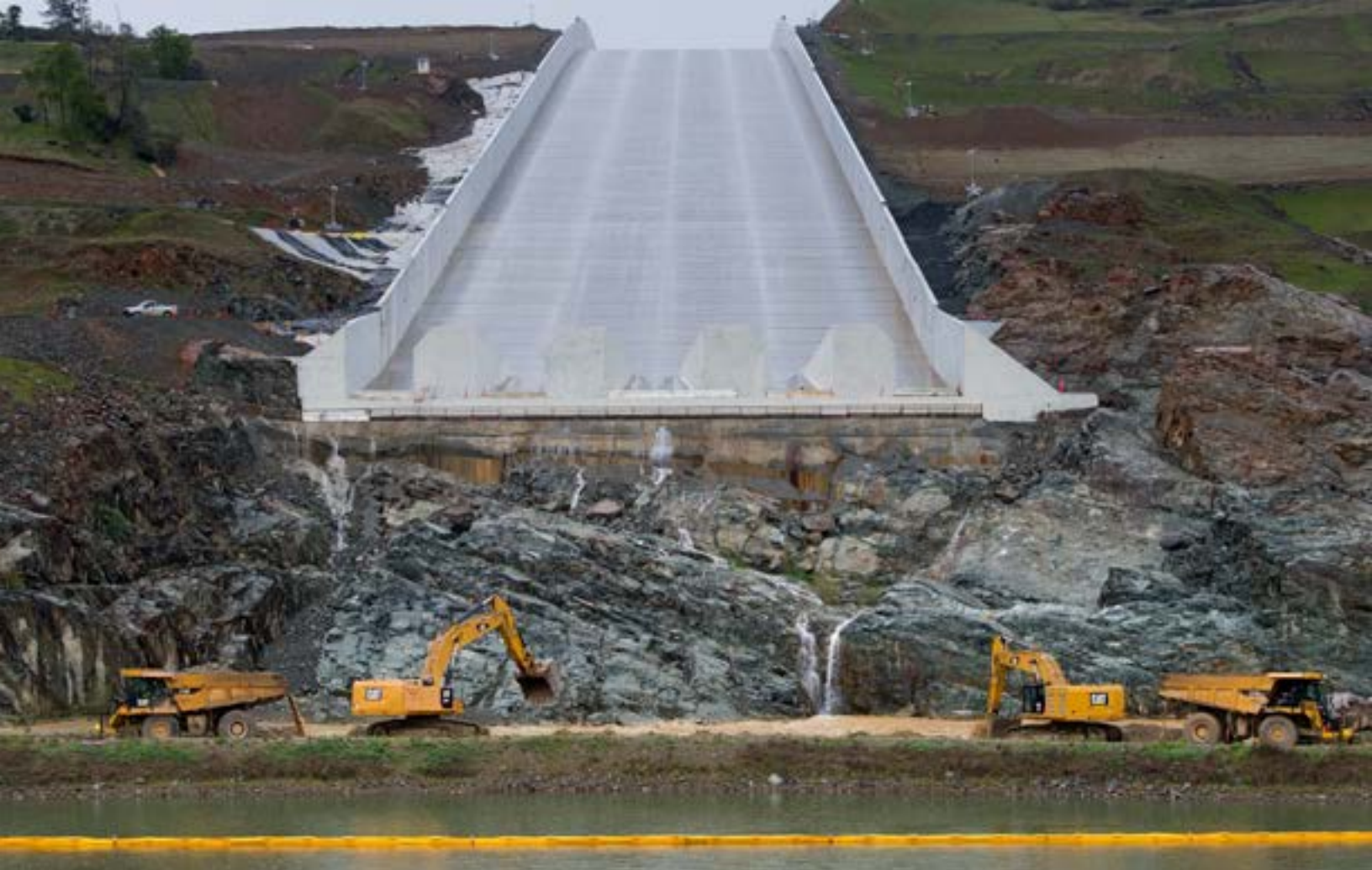
Oroville Spillway. Photo Courtesy of the California Department of Water Resources
